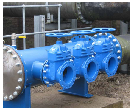
Manifolds Fabricated and Installed
