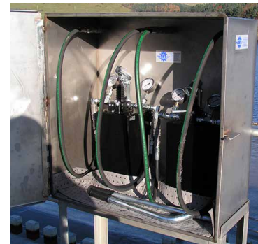
Multiple Penstock Hydraulics
